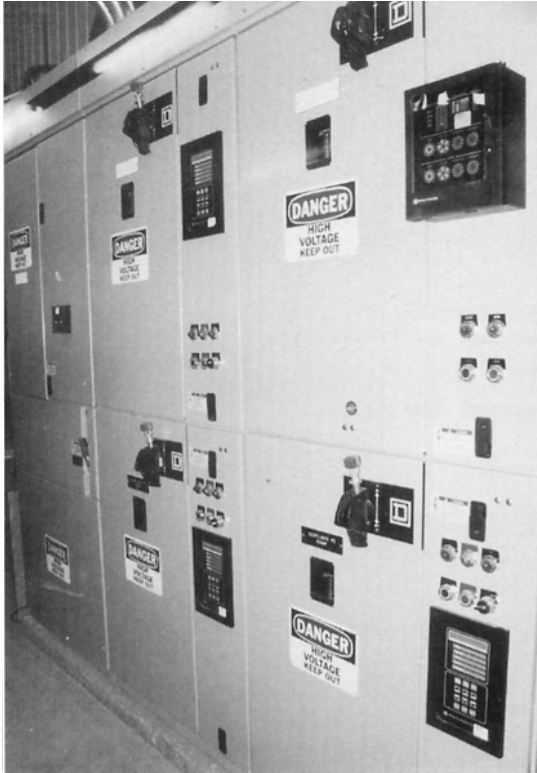
Figure 31.20 This 600-V, 3-phase motor control center is equipped with PowerLogic® devices that provide sophisticated monitoring capabilities such as active and reactive power, voltage, current, and waveform analysis. It includes Internet transmission capabilities and possesses embedded Web pages. (Courtesy of Schneider Electric)
